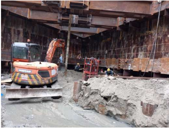
Figure A3: Excavator was switched off when it was not in use
