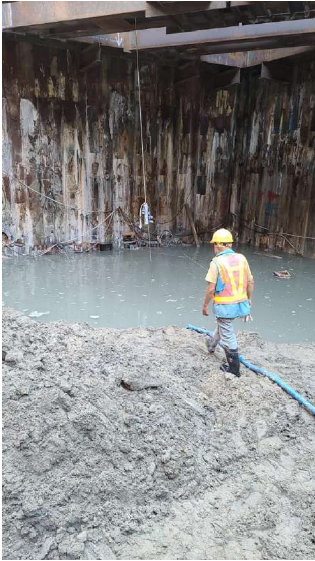
Figure A1: Water seepage at the cofferdam of ventilation adit in Portion 1D
